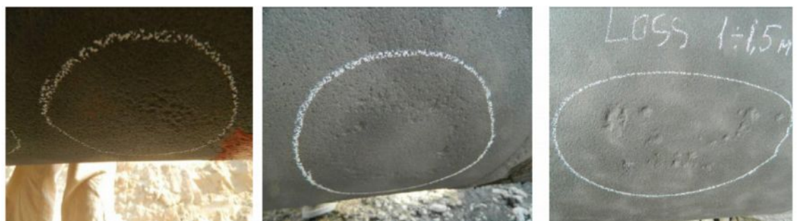
Fig. 3 Plots of pitting corrosion, the detected by indirect examination method in the buried pipeline. The depth of the buried pipe trench is 4 m.
