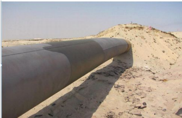
Fig.1 Violation of the geometry of the segment of buried pipe that caused the stress strain state at a critical level.
