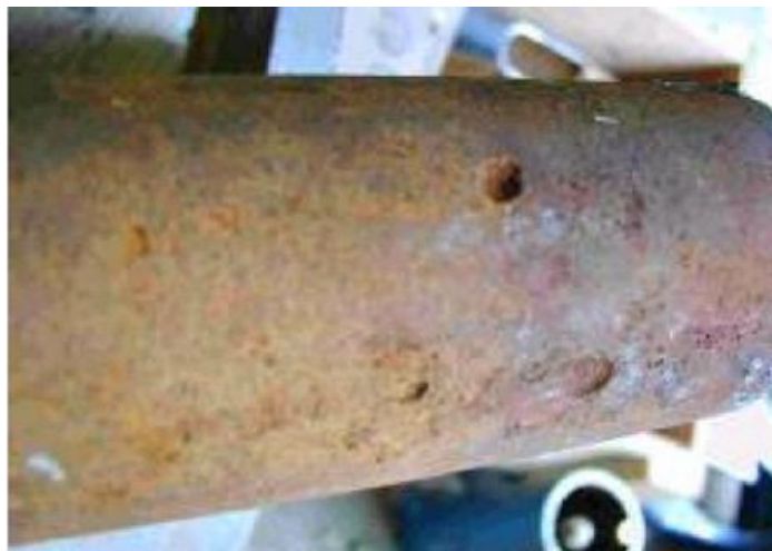
Fig.2 Plot of pitting corrosion, detected by indirect examination method in the segment of buried pipeline.
